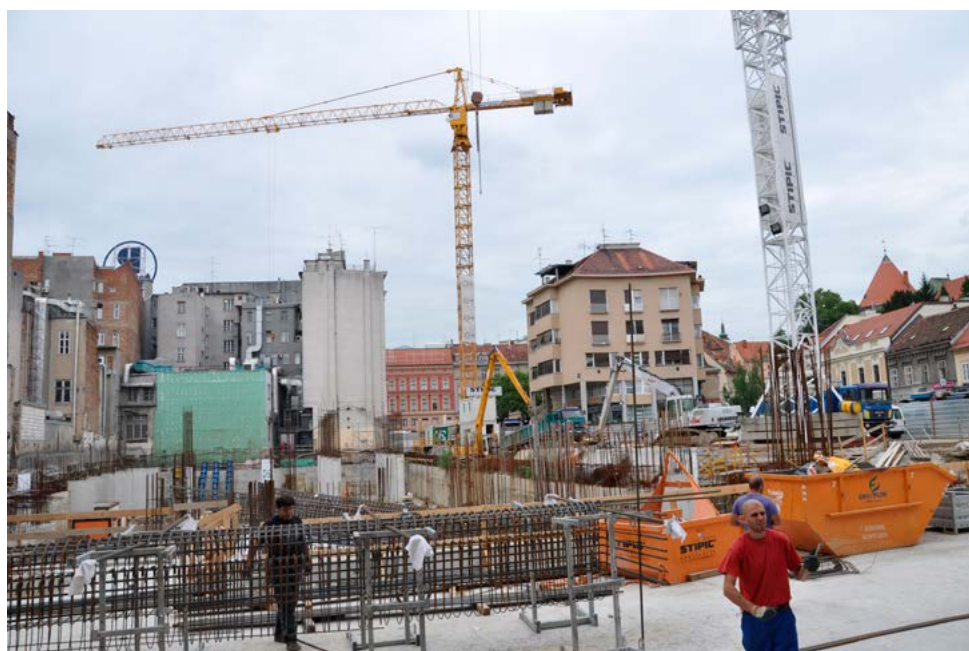
The construction of Ban centar , Zagreb, July 2011 (Portal of the Croatian Cultural Council).
