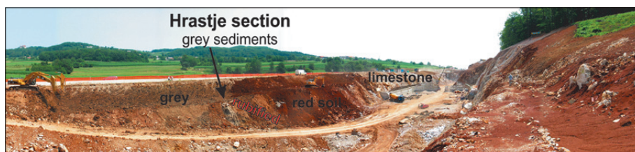
Fig. 2: Construction of the highway north of Novo mesto has exposed laminated grey sediments, which were surrounded by red soils developed on subcutaneous karst relief.
