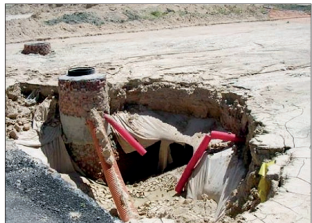
Fig. 12: Damages to a collector caused by broken pipes.
