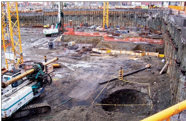
Fig. 14: Crater formed by the collapse of a pile in karstified gypsum.
