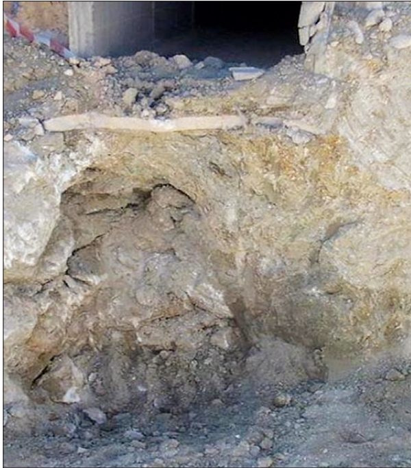
Fig. 13: Damage to collector caused by broken water pipe.
