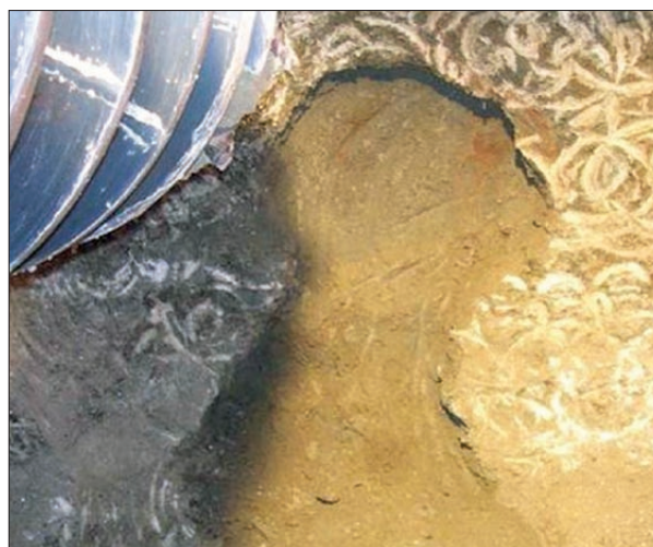
Fig. 9: Cavities formed by Karstic duct clogging by silty and clay deposits.
