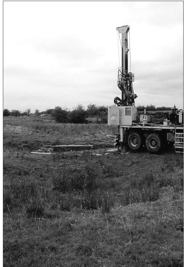
Fig. 5: Bedrock core drill rig in a dry valley, Mewlaghmore, Castlereagh. Note small closed depressions (Photo: C. Hickey).
