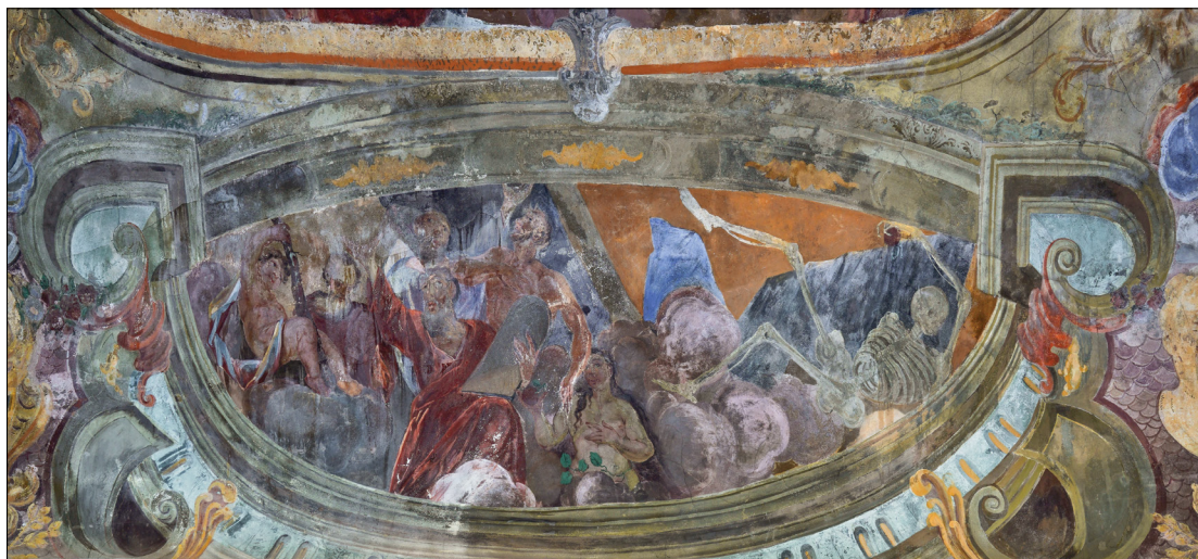
30. Southern section of the ceiling painting, Our Lady of Sorrows chapel, St George's church, Ptuj
