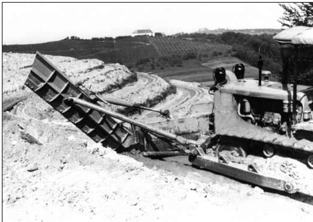
Figure 4: A bulldozer with equipment for creating terraces; Železne Dveri Mansion in the background (photographer unknown, Ptuj Historical Archives, collection: SI_ZAP/0255 Agrotransport Ptuj 1957–1997, box: 18).
