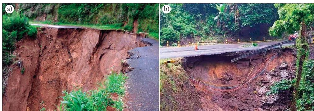
Figure 2: a) Example of a shallow landslide causing road collapse along the Jember–Banyuwangi route in the Gunitir Mountain Area, and b) damage to road infrastructure, including guardrails and exposed utility cables, following a landslide event.
