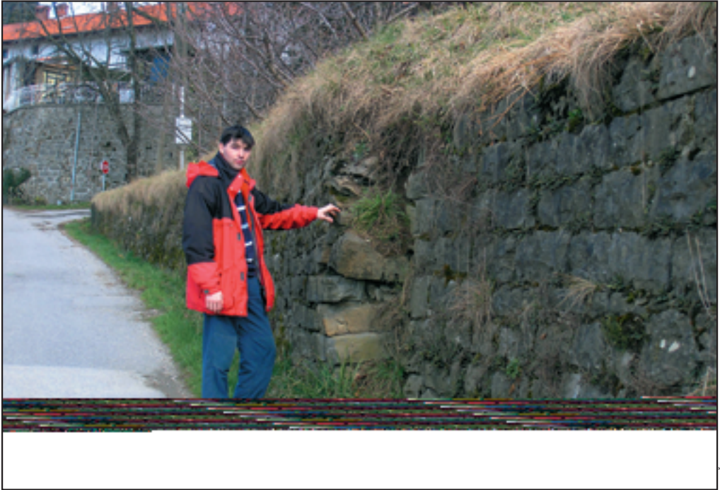
Figure 2: Bulging stone walls lining road cuts due to landsliding.
