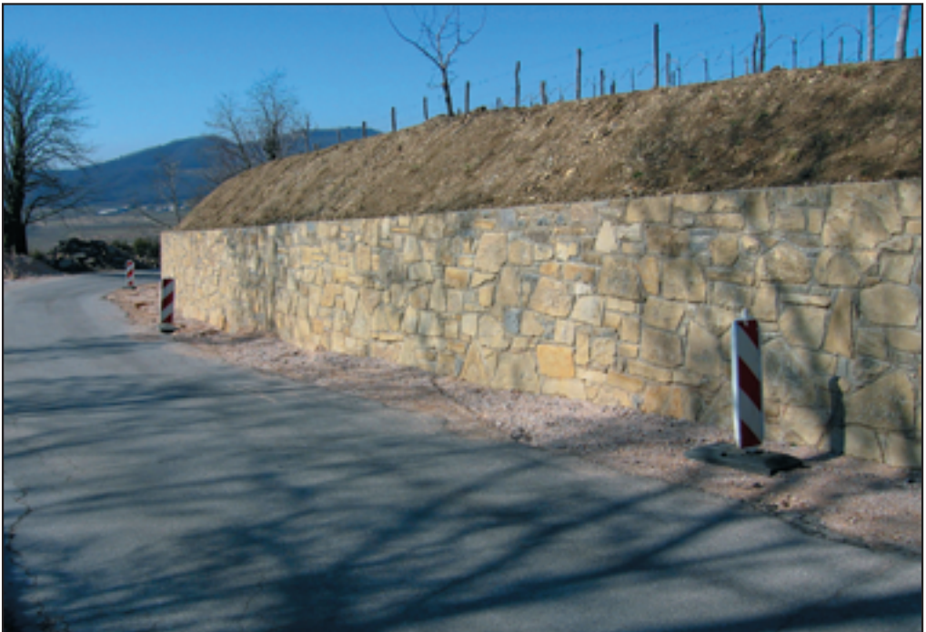
Figure 3: Stone walls require constant maintenance due to landsliding.
